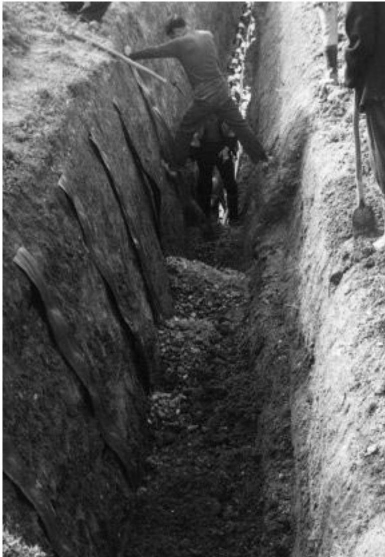
Dam seepage project in China
