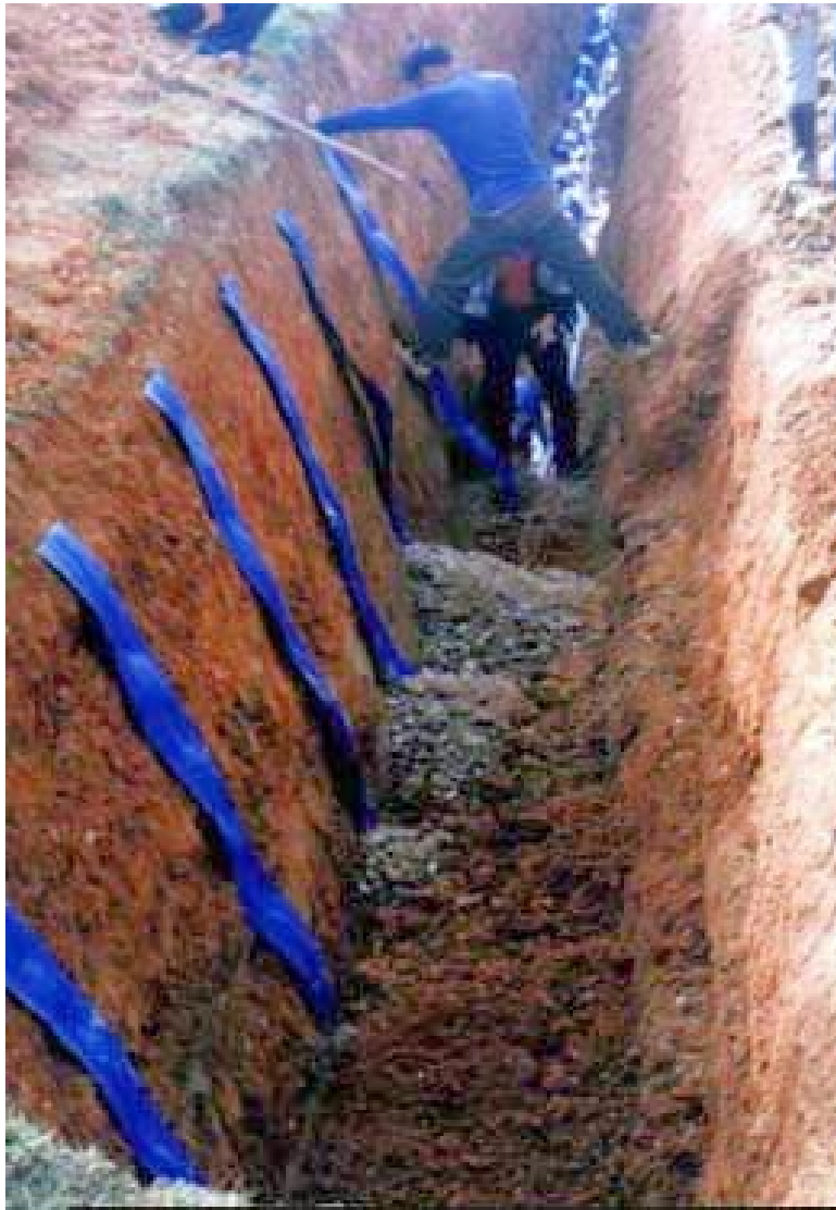
Dam seepage project in China
